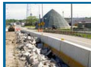
Workers removed the median curb as part of preliminary work to rebuild the flyover bridge over the Northwest Tollway to U.S. 20.
