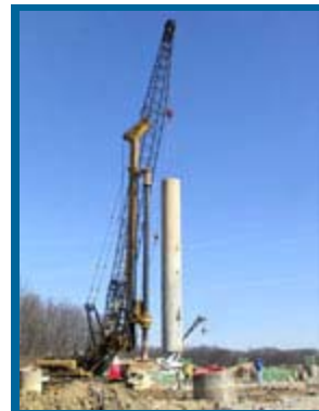
A 100-foot long steel liner is placed in the ground for the foundation of the new Des Plaines River Valley Bridge north of Bluff Rd.
