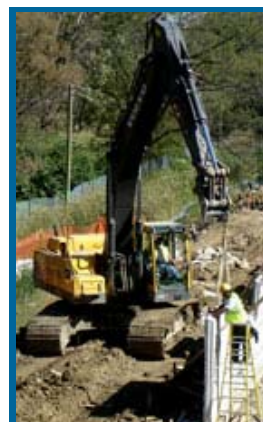
Panels are set for a retaining wall along I-88 as part of the advance work for a rebuild and widen project from Washington Street to Finley Road
