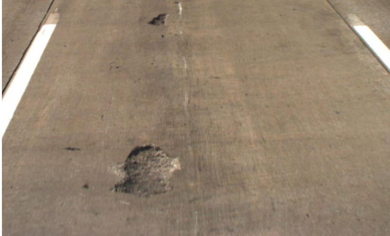
Figure 23. Example of distress that requires partial-depth repair.
