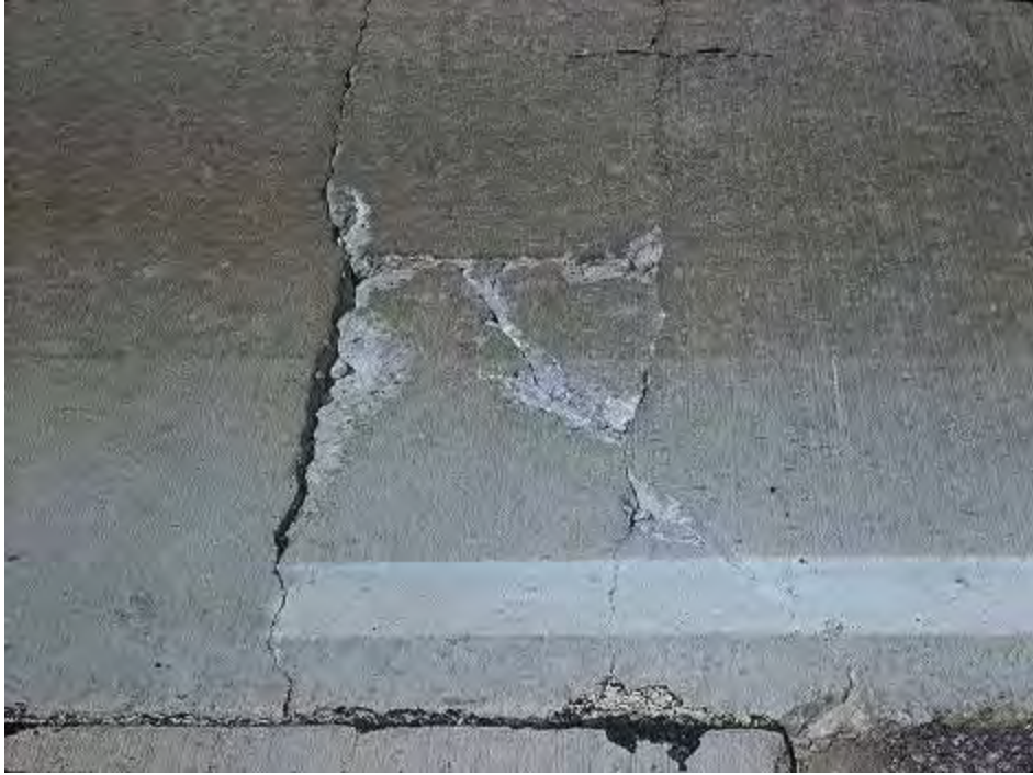
Figure 22. Edge punchout on CRC pavement (Gulden, 2013).
