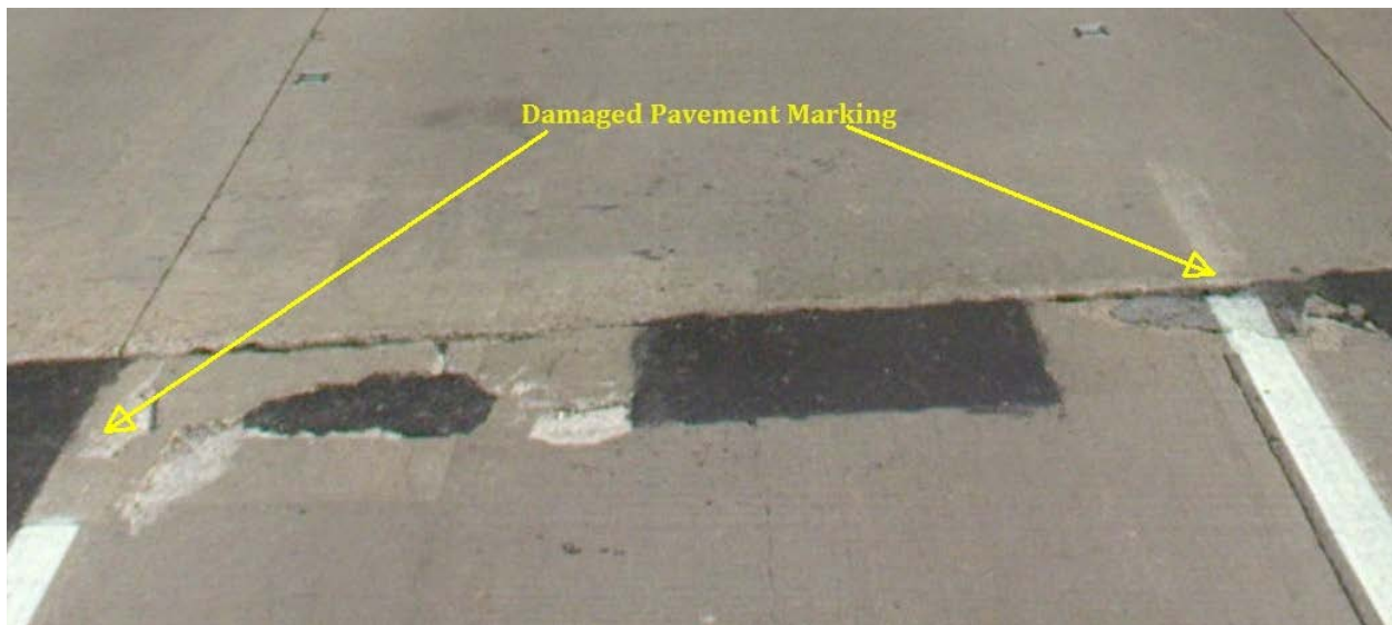
Figure 8. Damages lane mark by pavement distresses.
