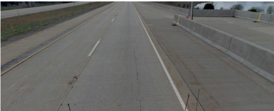
Figure 14. Moderate-severity longitudinal crack.
