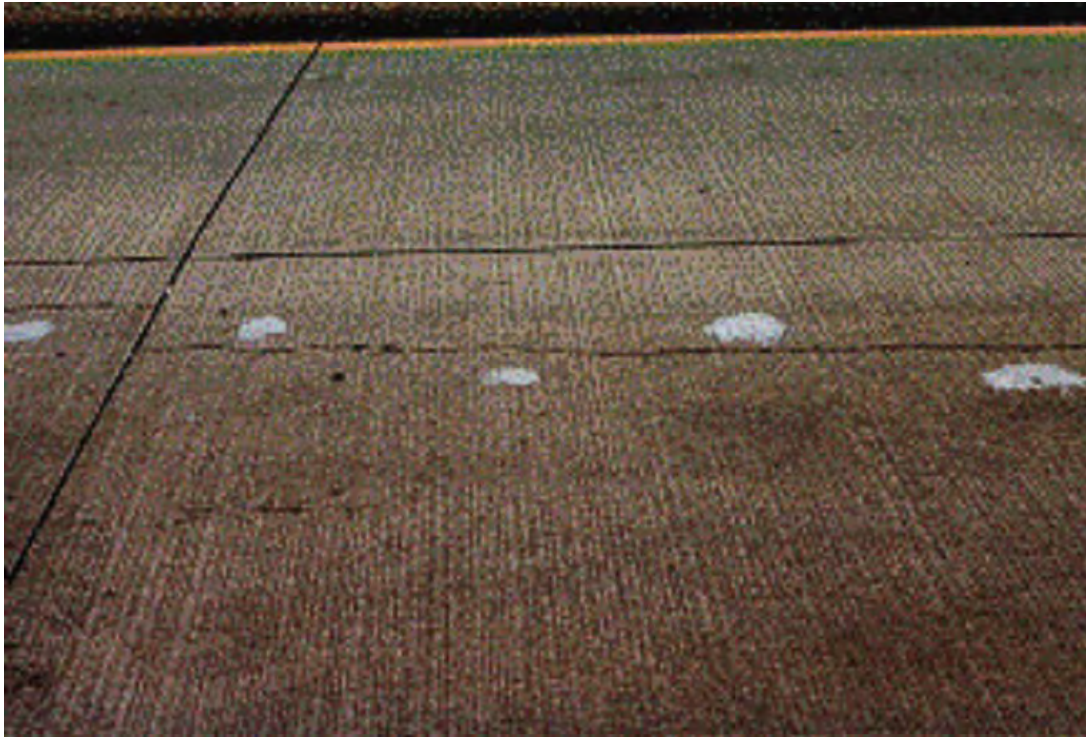
Figure 26. Example of cross-stitching to control longitudinal crack in jointed plain concrete pavement (IGGA, 2010).
