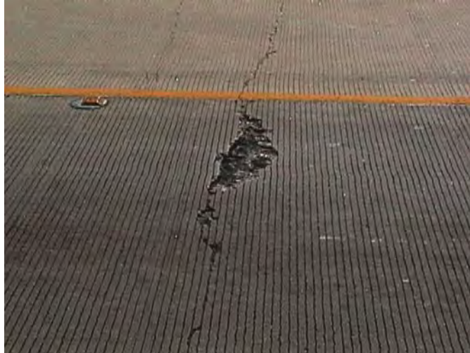
Figure 19. Spalling along transverse crack ( http://crcpavement.org ).
