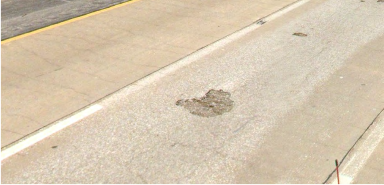
Figure 11. Surface distress on CRC pavement.
