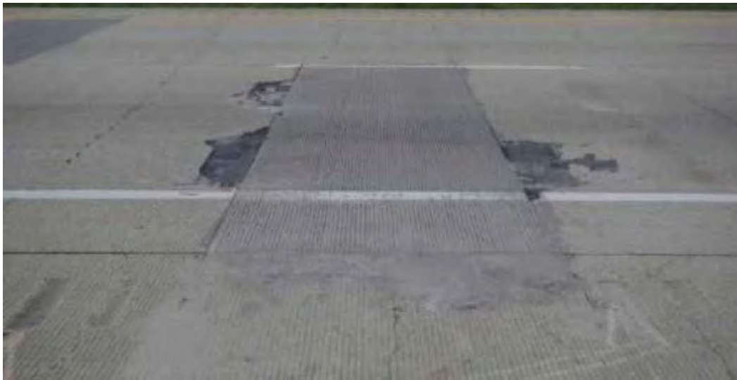
Figure 29. Punchout at repair joints (Ryu, Choi, Choi, & Won, 2013).
