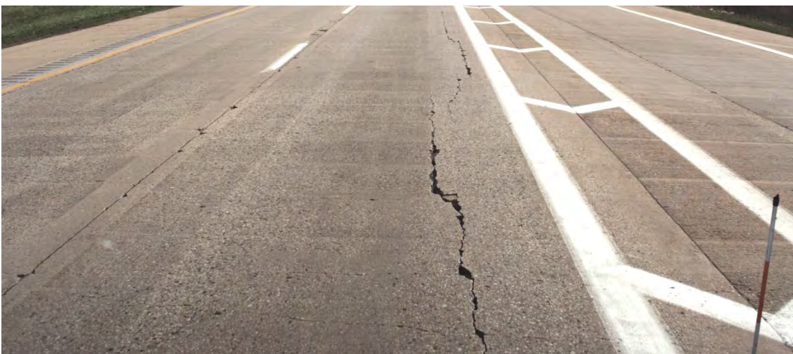
Figure 15. High-severity longitudinal crack.
