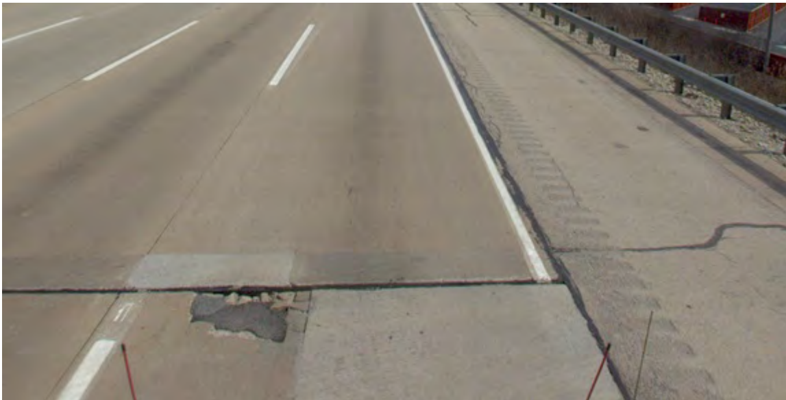
Figure 21. Punchout at the construction joint.
