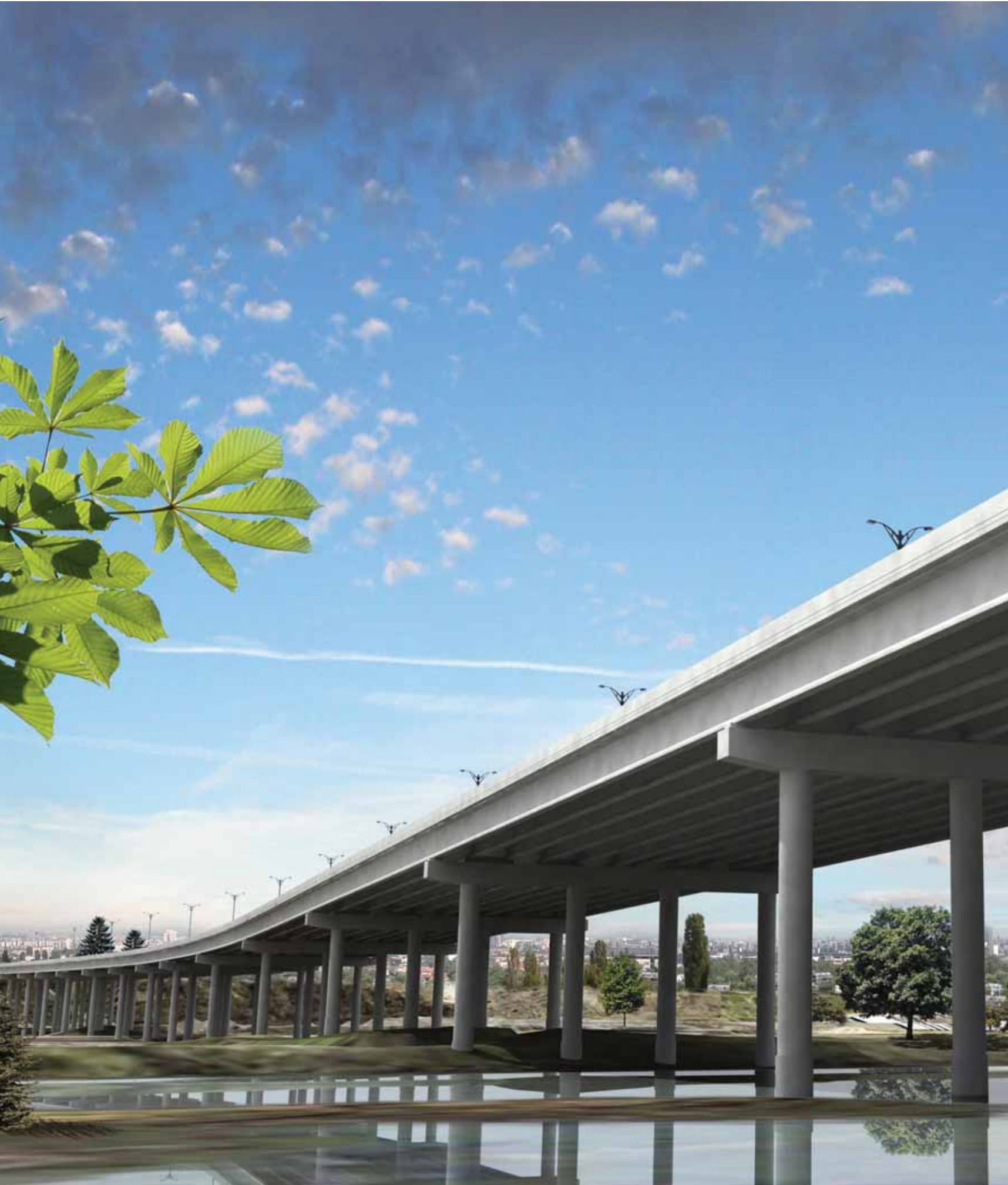
THE 1.3-MILE DES PLAINES RIVER VALLEY BRIDGE on I-355 South will be the longest on the Tollway system.
